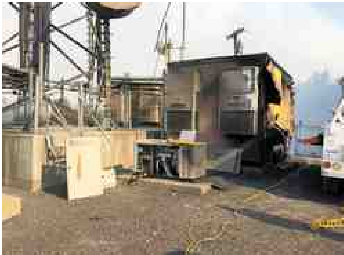
California wildfires: Telecoms infrastructure damage.
